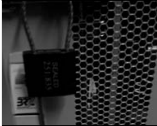
Figure 4: Sealed security rack
